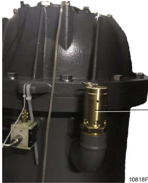
Location of safety valve on air-cooled compressor
