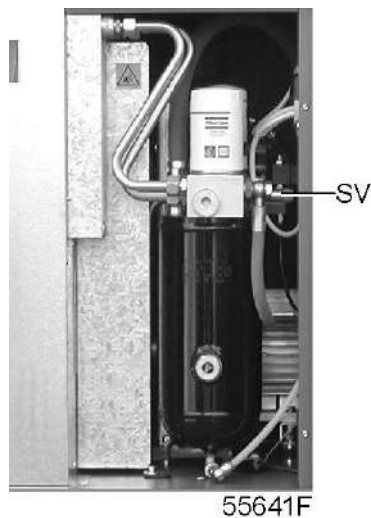
Safety valve on the compressor
